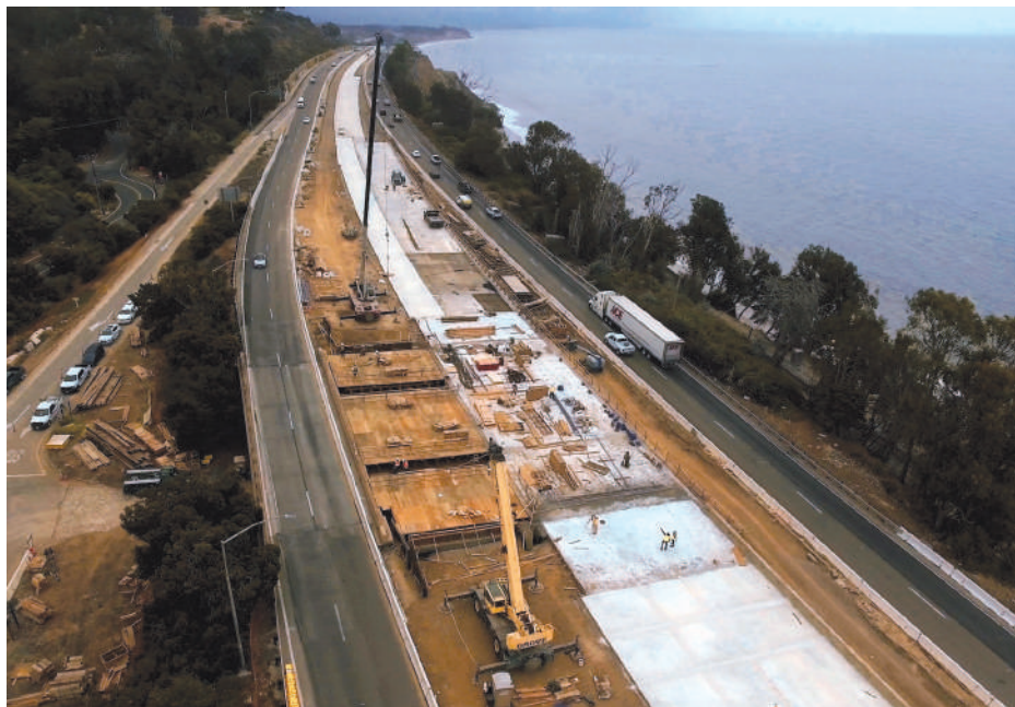
RELIEF Granite is serving as construction manager for the U.S. Route 101 upgrade, including new carpool lanes.
